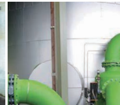
CPP(Condensate Polishing Plant)
